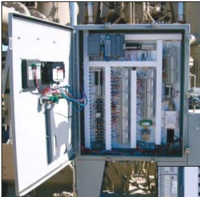
■ The Remote Operations Management (ROM) panel for integrated compressor monitoring, control and diagnosis developed by The Hanover Company Four Corners Region Instrumentation and Electrical (I&E) team. Note the M2M intelligent iGateway module in the inset photograph.
