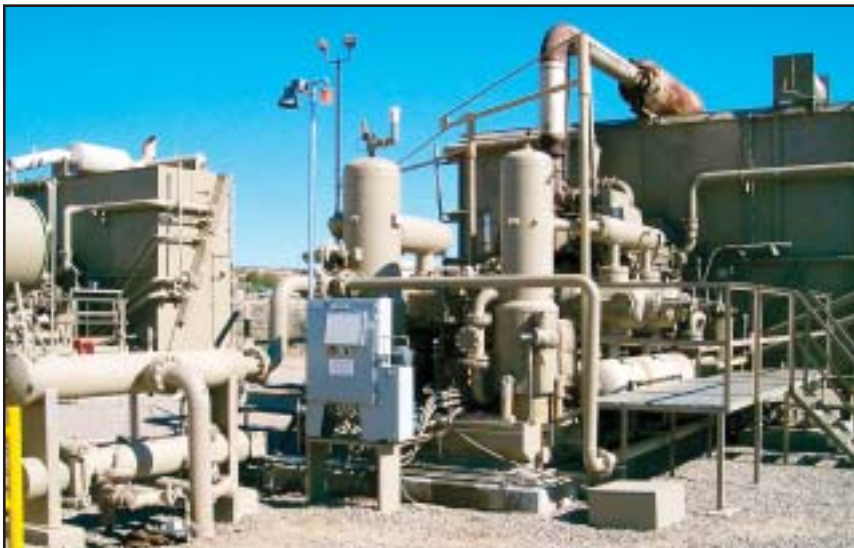
■ The Hanover Company operates more than 600 high-value compressors for Williams Field Service near Farmington, New Mexico, U.S.A.
